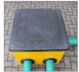
Electrical Draw Pits
