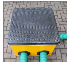
Electrical Draw Pits
